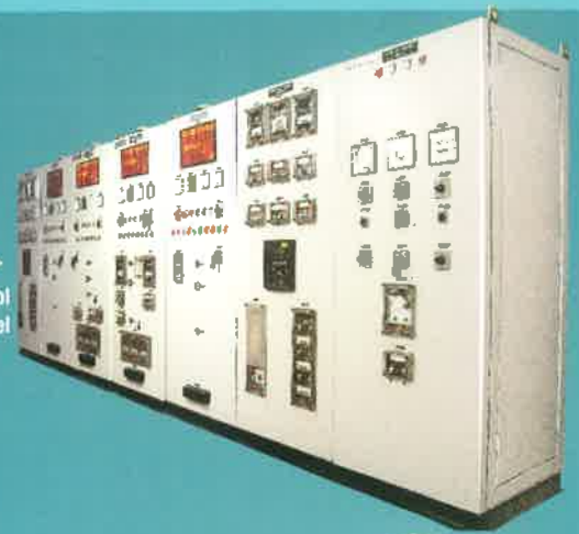
Control & Relay Panel
